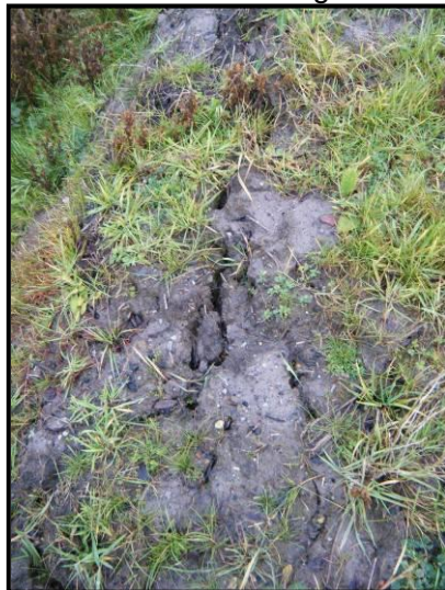
Cracking in upper surface of embankment
