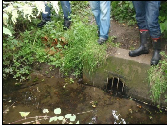
Original storage pond inlet (Right) with new Environment Agency triple pipe inlet (Left)
