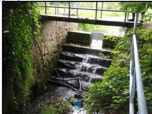
Stepped outfall from storage pond
